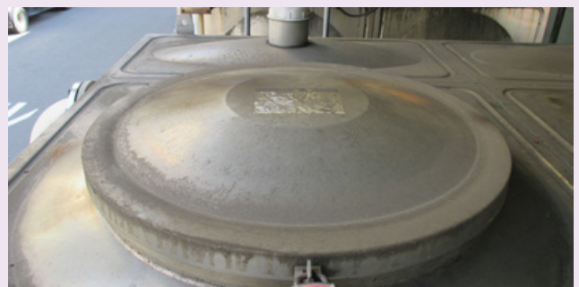
Locking of a process-water tank outside the production area
