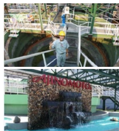
Top: Wastewater treatment equipment at Bien Hoa Factory Bottom: Waterfall monument installed beside wastewater treatment equipment
